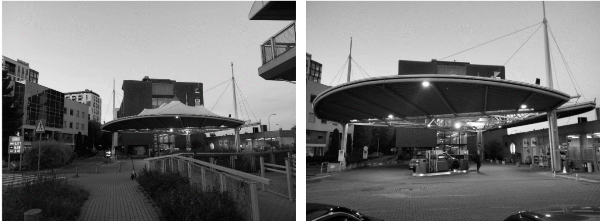
Fig. 5, Fig. 6. Structural system of the roof covering, varied with combinations of steel trusses at a gas station for cars in Gdynia.
