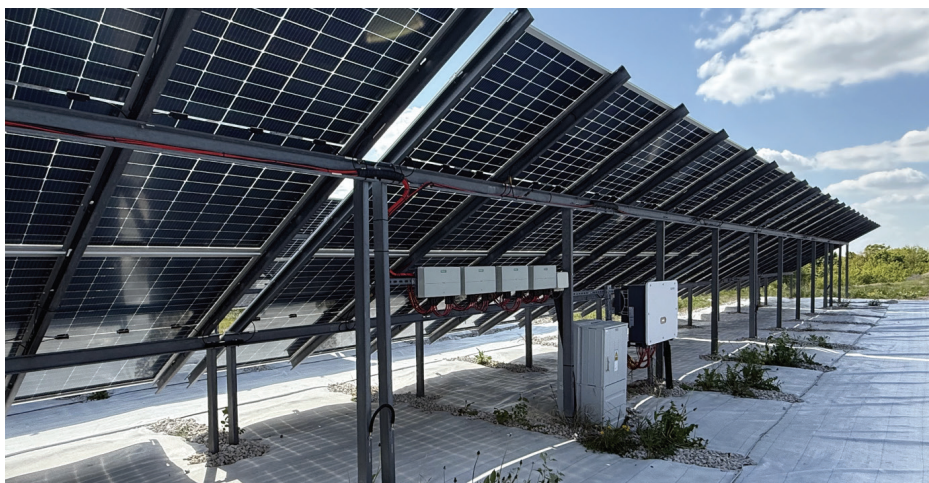
Fig. 1. Ground-mounted PV installation on the reclaimed Zakroczym landfill.
